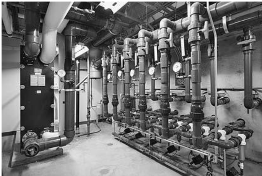
Figure 5: Geo-Exchange Water Pipes and Manifold in the Friends Center's Mechanical Room, Philadelphia
