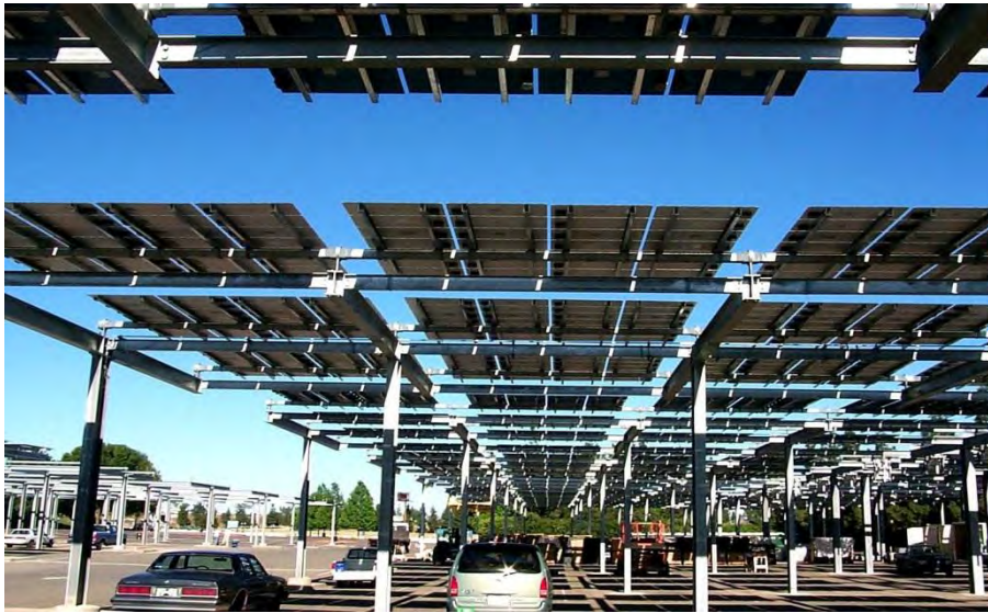
Figure 45: Elevated photovoltaic racking structure for 540kW system
