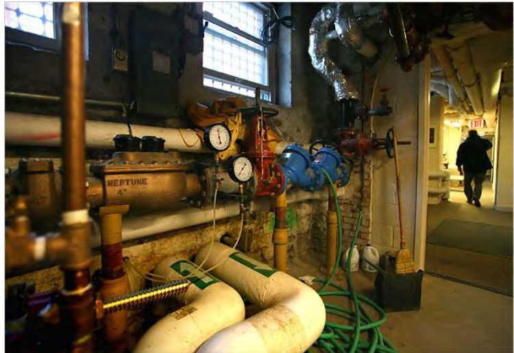
Figure 21: Geo-Exchange Water Input and Return Pipes in the Basement of Chelsea General Theological Seminary
