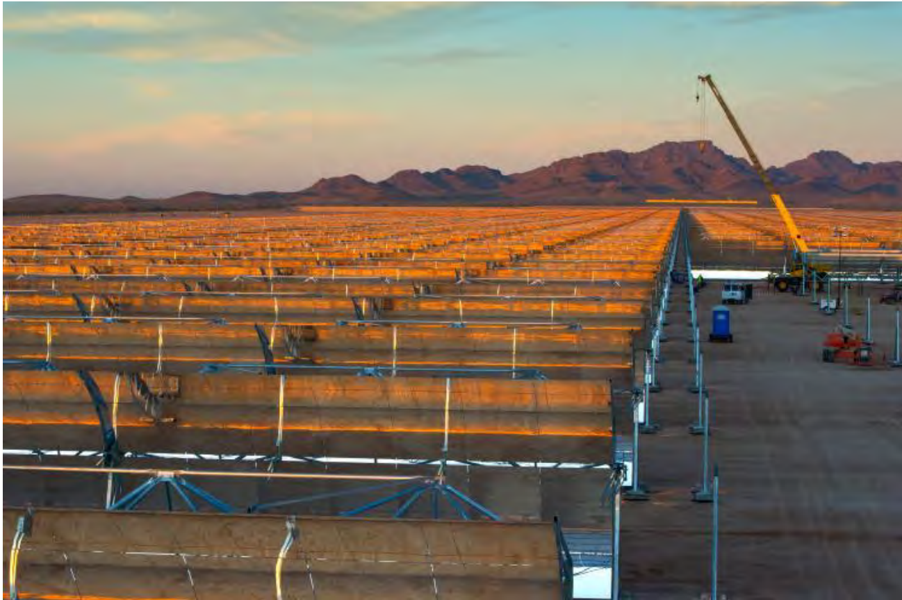
Figure15: Concentrating Photovoltaic Solar Array in Gila Bend, AZ
