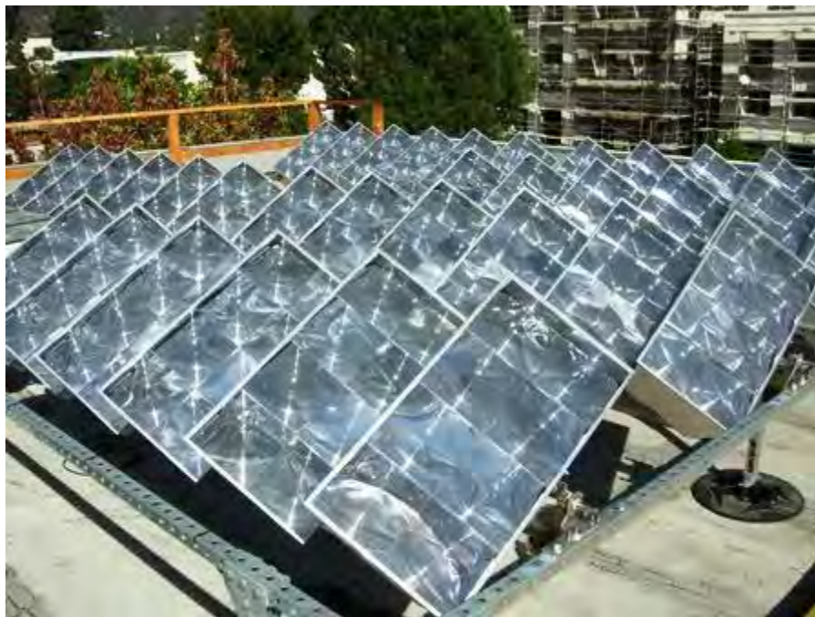
Figure 4: Emcore Soliant 1000x high-density rooftop CPV
