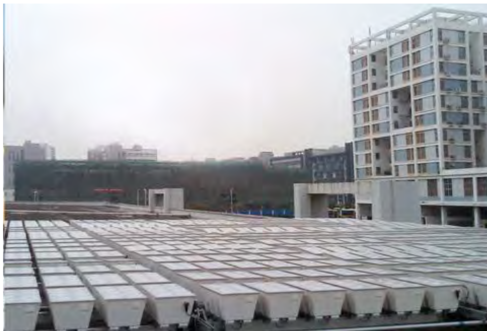
Figure 51: Rooftop CPV installation
