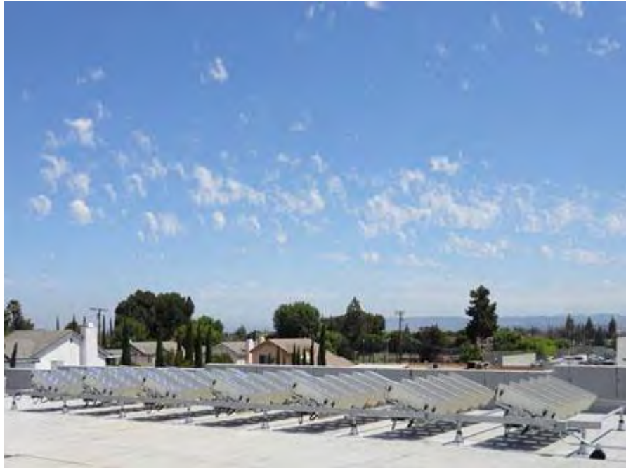
Figure 52: Tracking CPV rooftop racking system
