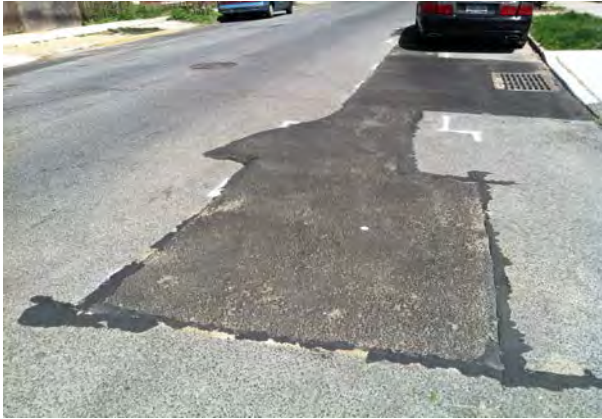
Large area of asphalt patches on the road and around catch basin.
