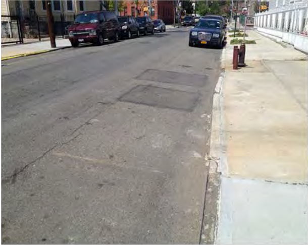
Utility poor repave
