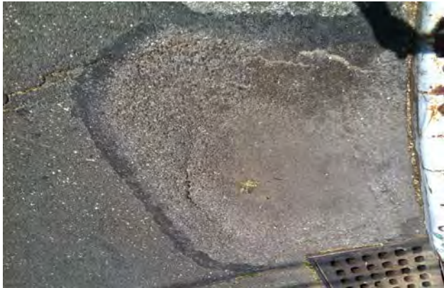
Re-pavement and deterioration of the asphalt
