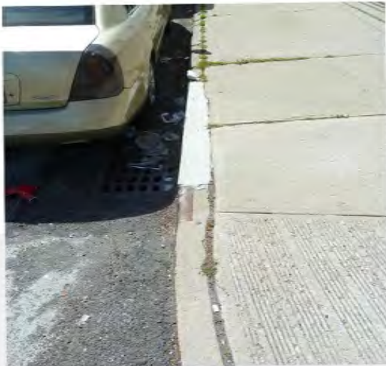
Catch basin with a lot of trash
