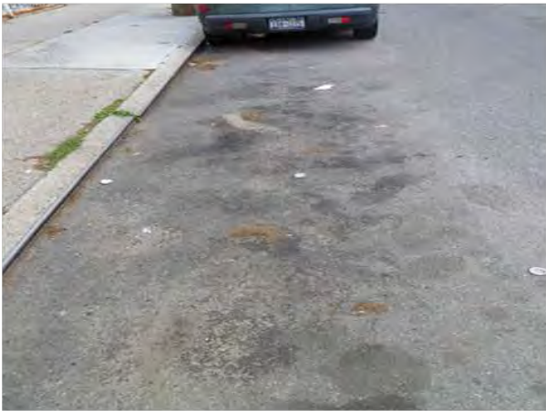
Worn down pavement
