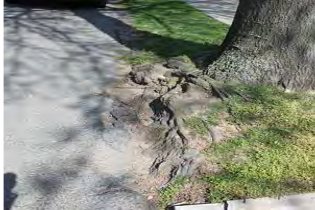
Tree roots impeding on roadway
