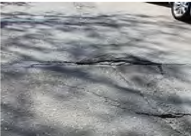
Big cracking and damage on the asphalt.
