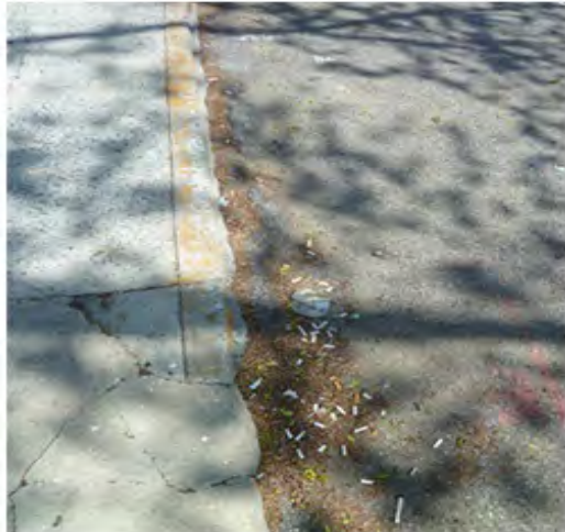
Cracking sidewalk and broken gutter
