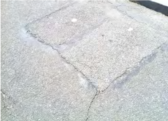
Cracking and patches of the asphalt.
