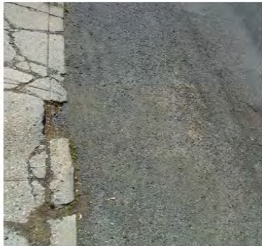
Missing curbs and raveling surface
