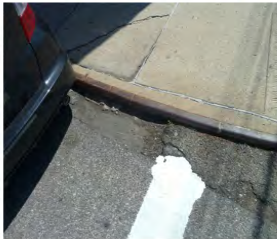
Newly painted pedestrian crossing line and broken asphalt
