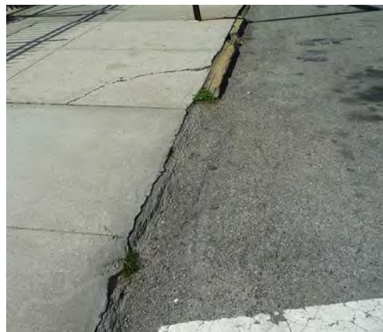
Missing curbs around the driveway sign.
