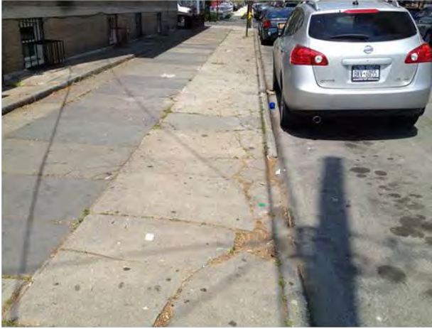
Old sidewalk and roadway
