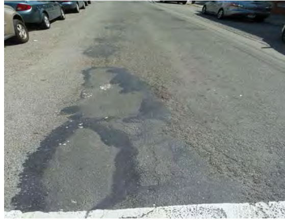
Patches on the broken asphalt.
