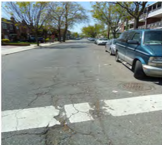
Cracking and holes through crossing lines and manhole
