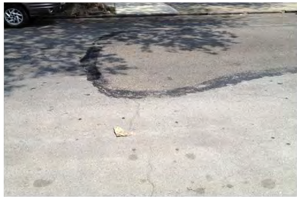
Utility uneven repave
