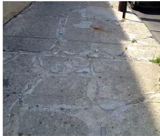
Severe cracking on sidewalk
