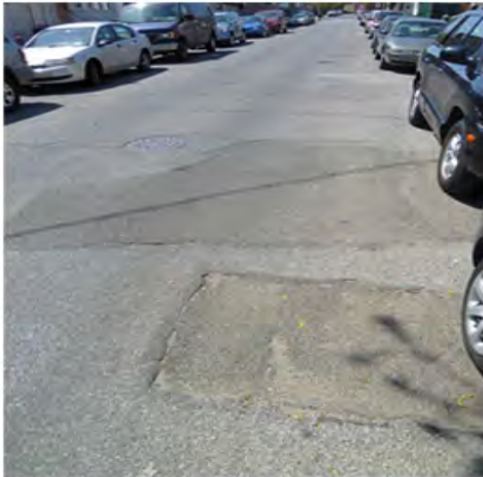
Repavement and patches of asphalt
