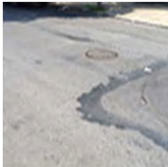
Pothole near manhole cover
