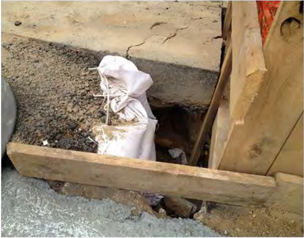
Holes due to construction
