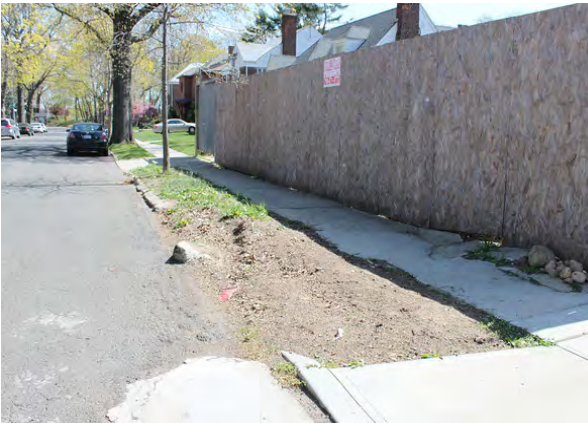
Sidewalk damage from adjacent construction
