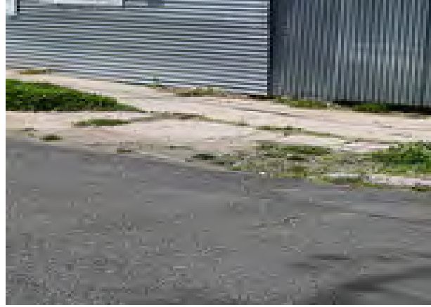
The broken sidewalk and curbs with weeds in the cracks.
