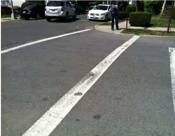
Faded pedestrian crossing line and uneven pavement
