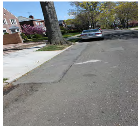
Gutter lane in need of repair
