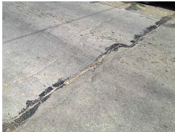
Large cracks in roadway
