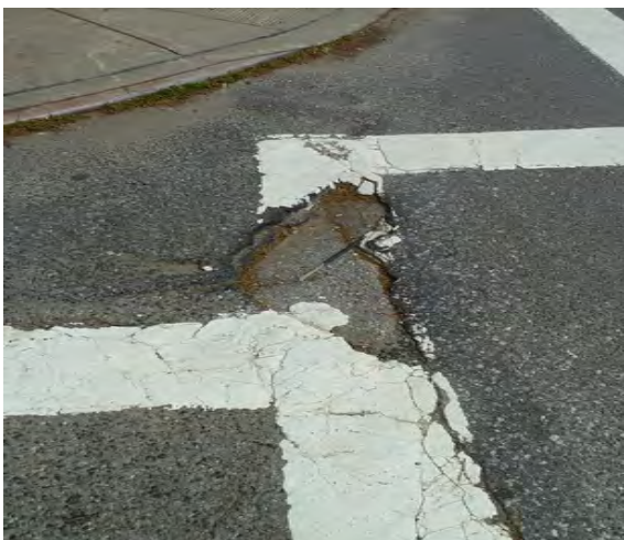
Cracking in x-walk
