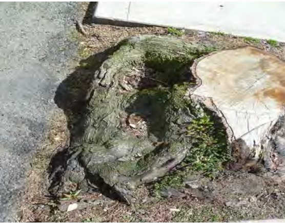
Missing curb and a dead tree.
