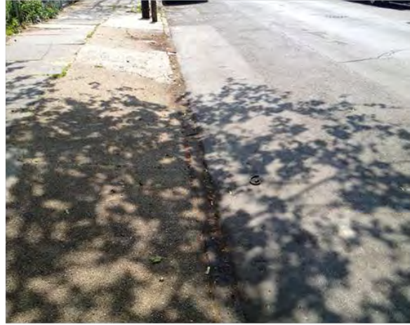
Sidewalk cracking near roadway surface
