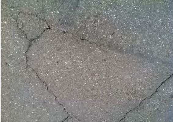
Cracked asphalt on road surface.
