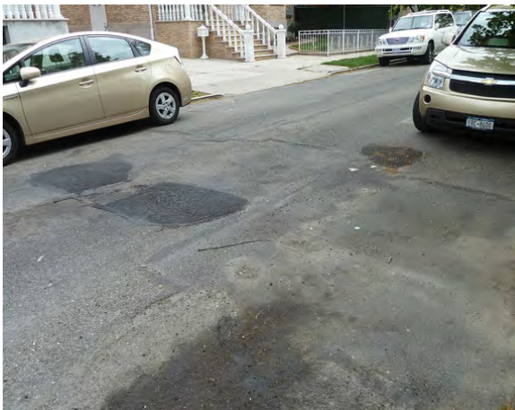
Pavement patching and cracking
