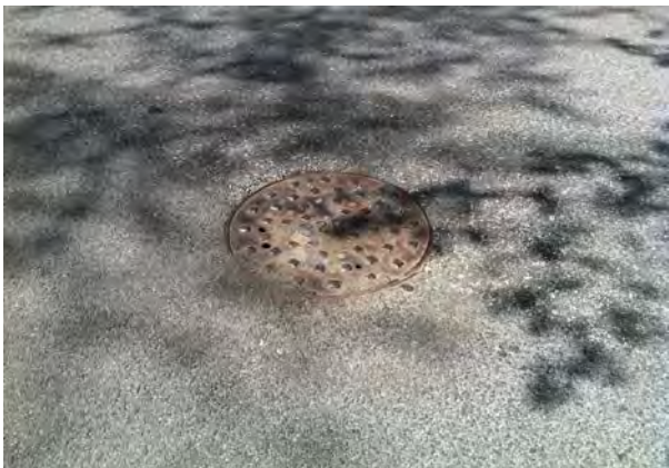
Abandoned manhole sealed into the ground.
