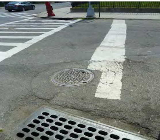
Patches and cracking surrounding the manhole and catch basin.
