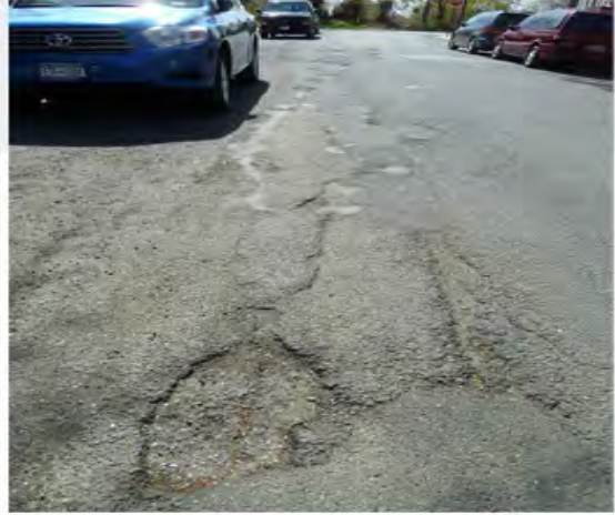
Potholes and cracking of asphalt
