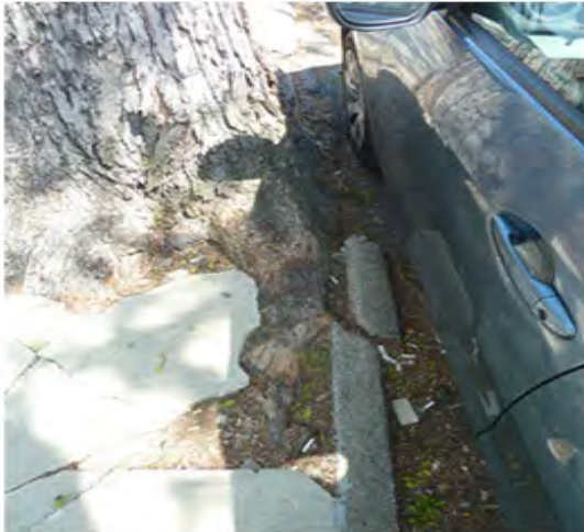
Broken curb due to tree roots and parking
