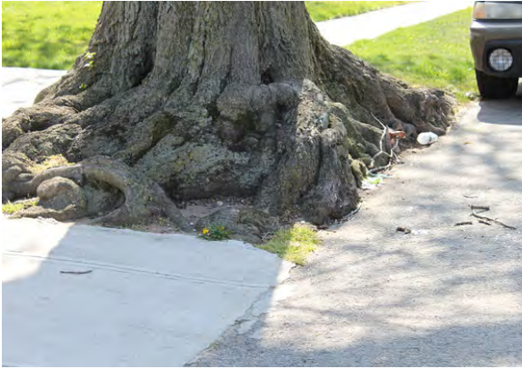
Tree roots impeding on roadway
