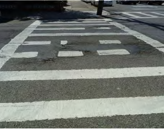
Cracking and holes on the crosswalk.
