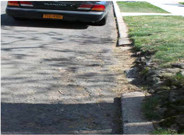
Tree roots impeding on roadway
