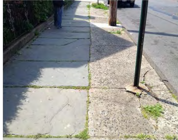
Sidewalk cracking near roadway surface
