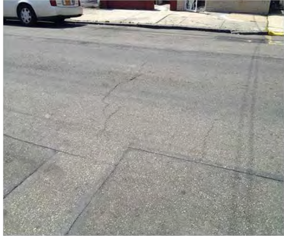
Cracks in roadway
