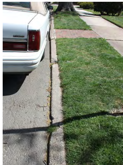
Cracked curb in need of repair
