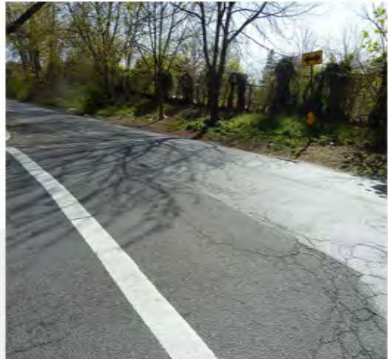
Cracking asphalt with no curbs at all
