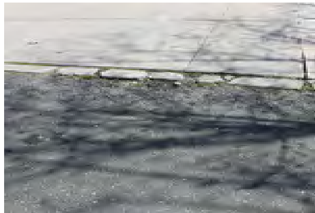
Segmented curbs and raveling asphalt surface.
