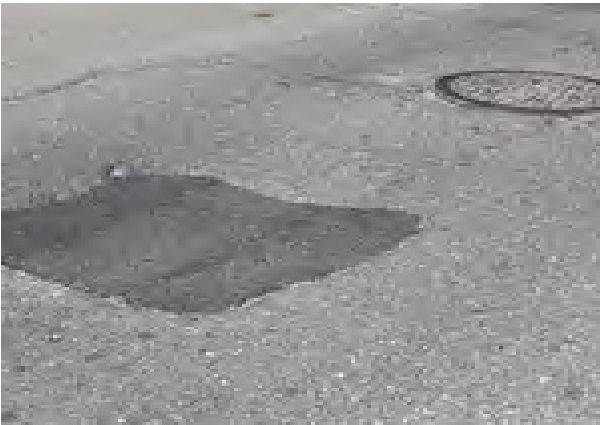
Cracking and patches of the asphalt.
