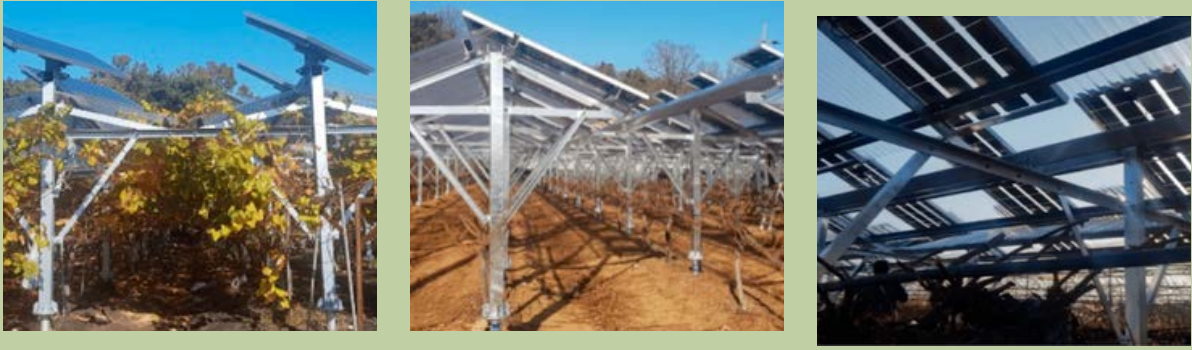
Figure 4. Installation of three different types of solar panels from left to right: normal, bifacial, and transparent.
